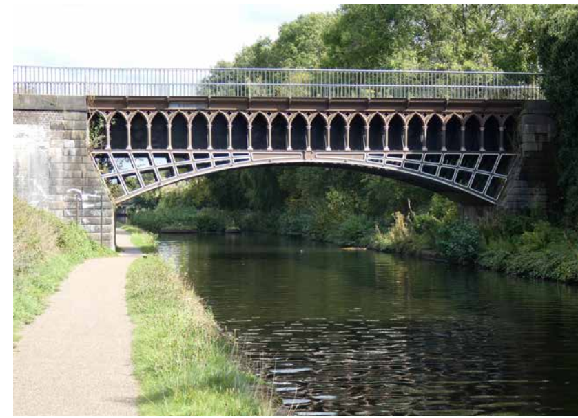
Engine Arm Aqueduct from the New Main Line (Grade II* listed, SM)
