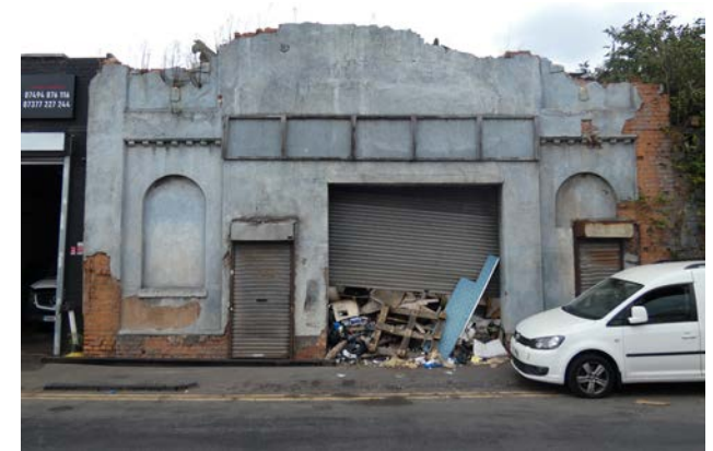
Plate 2.36 Fire damaged premises at 74 Rolfe Street
