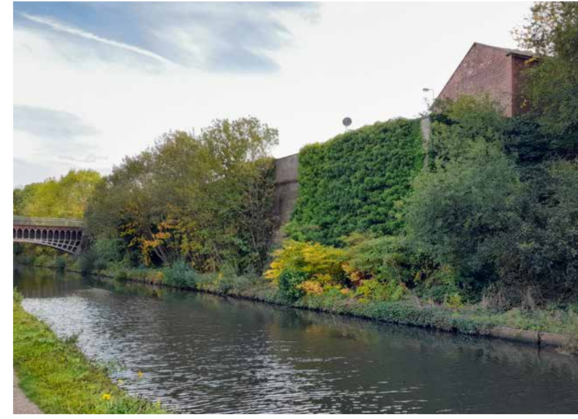
Retaining wall to the Corporation Yard along the New Main Line (Grade II listed)
